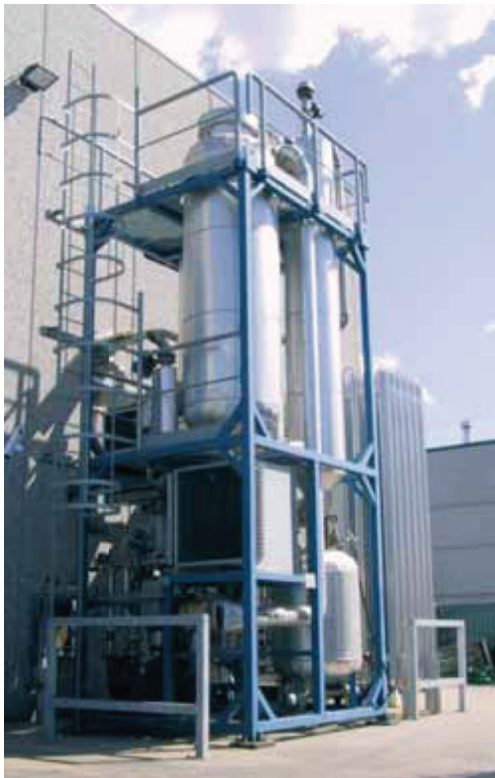
Figure 5: Cryogenic trap plant
